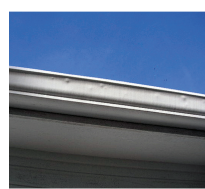
Damaged gutters, downspouts, fascia, Do a thorough inspection by walking around the property.
