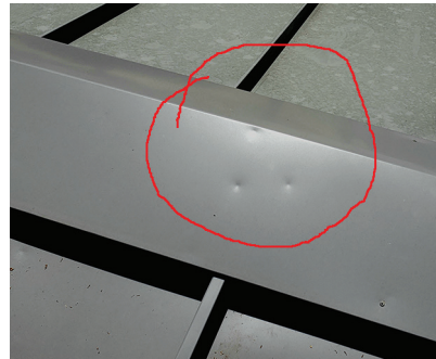
Standing Seam Damaged by Hail
