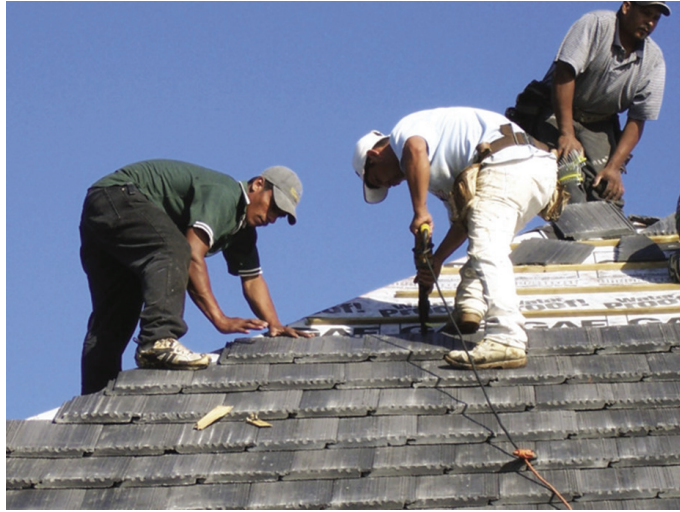
CR&R ltd installing a flat concrete tile roofing system, Proper installation consist of using proper fasteners, underlayment, batten boards, spacing, and mortar.
