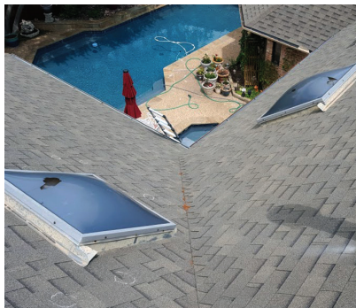
Skylight broken by hail
